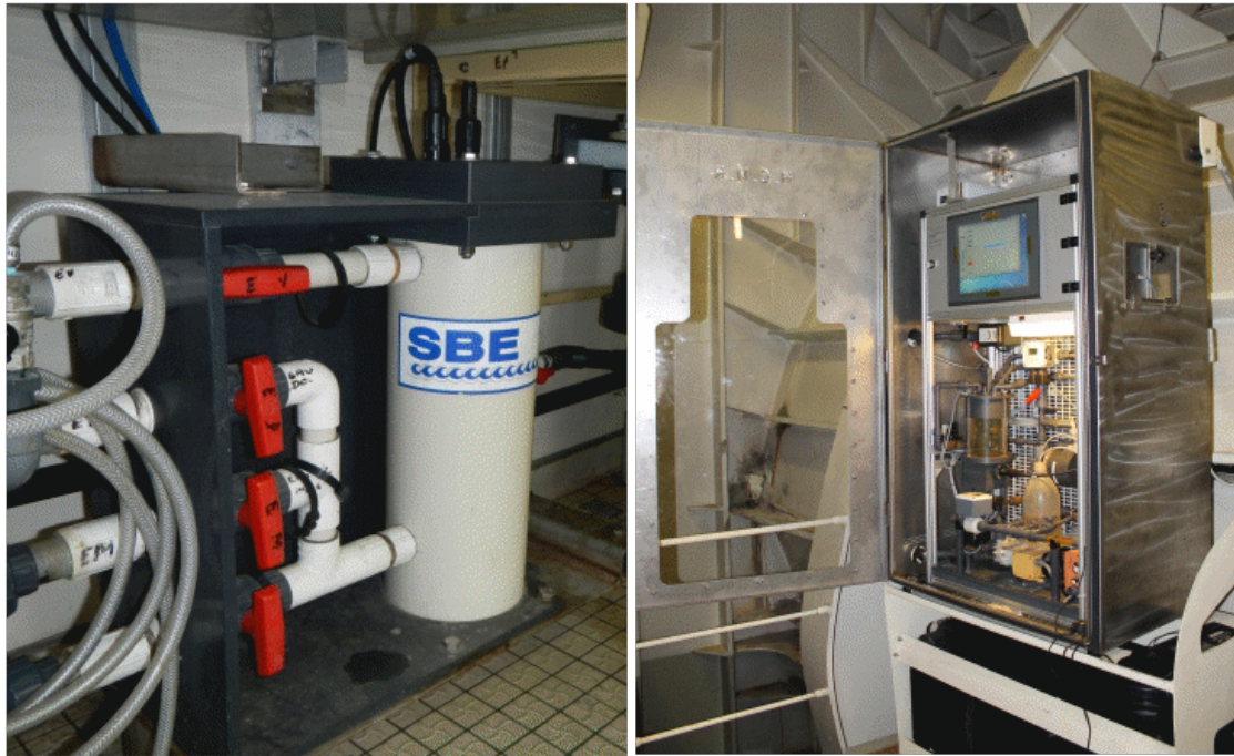
Figure 4. Thermosalinograph (on left) measures both SST and SSS. FerryBox (on right) is a flow-through system with multiple sensors for automatic measurements of several physical, chemical and biological variables.
